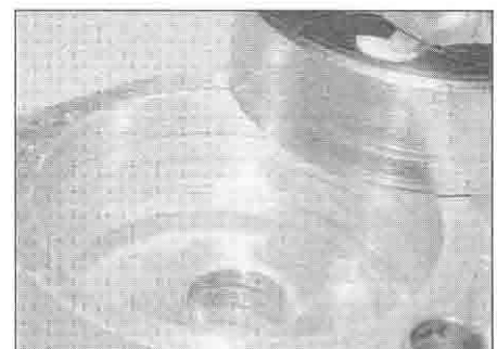
25.8 Scoring is evident on this pump rotor and in the housing
